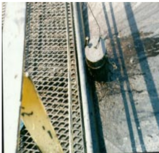
Photo of an unsecured sampling port hatch on a level 2 tank.
